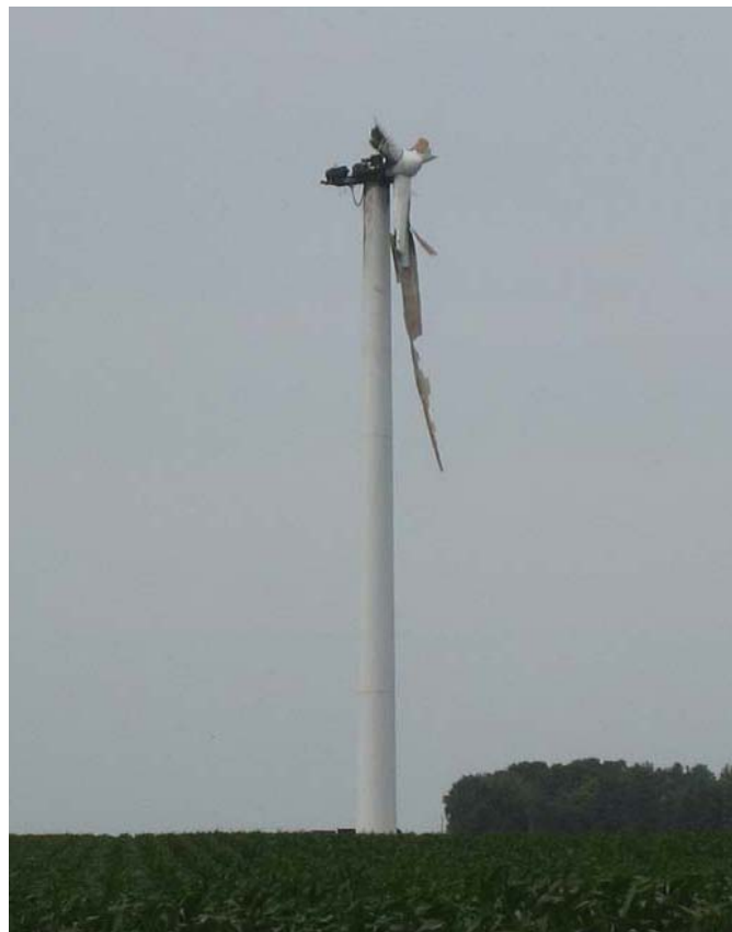
Figure 7. Lightning strike damage on a wind turbine in southern Minnesota, USA, resulted in the destruction of the nacelle and the rotor blades.
