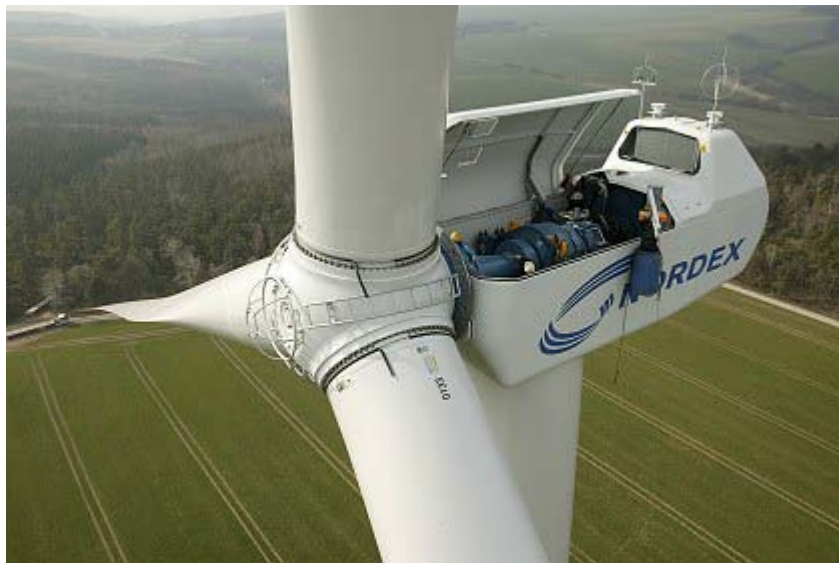
Figure 1. Maintenance at wind turbines nacelles involves work at about 100 meters height. Source: Getty, Nordex.
